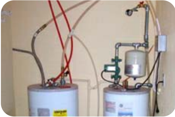
Heat Exchanger in Shed ©Melinda Honn
